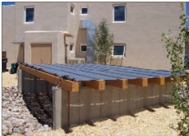
Figure 1. A night sky radiant cooling system installed in Taos, N.M. (Image courtesy of Cedar Mountain Solar, LLC.)
