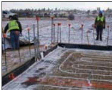
Figure 2. Hydronic tubing layout with HePex radiant on a cold winter's day.
