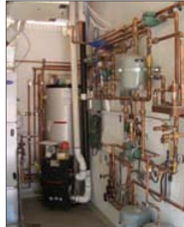
Figure 5. Hydronic heating system in mechanical room. Components include: Voyager 80-gallon stainless steel storage tank with condensing boiler gas back up for heat and domestic hot water; Taco circulating pumps (green pumps); Crown “brazed plate” heat exchanger CBP5X12-20 (foreground right); Laing PV-direct solar glycol circulator (small bronze and black/silver pump); Taco EBV zone valves (near the floor); ZVC control boxes and SR relay enclosures (green boxes); and Tekmar 155 and 152 differential and set-point controls (mounted on gray box).
