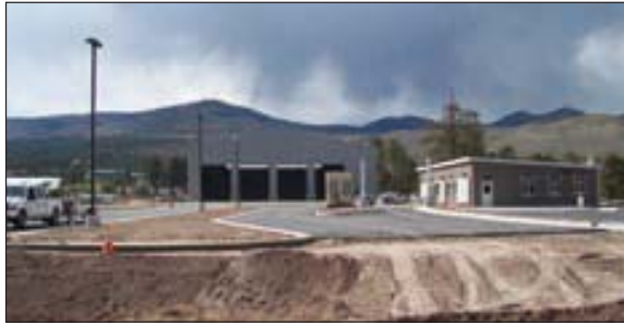
Figure 1, Waste Transfer Station Facility components include Viessmann Solar Collectors, Vitosol 100, flat plate, internal headers with vertical orientation and white shipping covers still in place.
