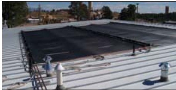
Figure 4. Roof of Eco Station features Heliocol HC-50 unglazed plastic radiator panels for cooling.
